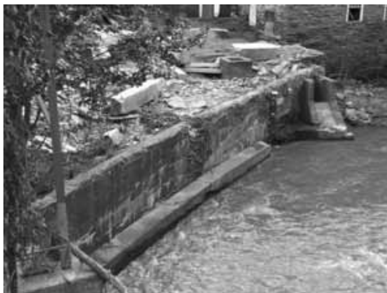
After: the Interpretive Area and retaining wall suffered severe damage by the flooding Mill Brook
