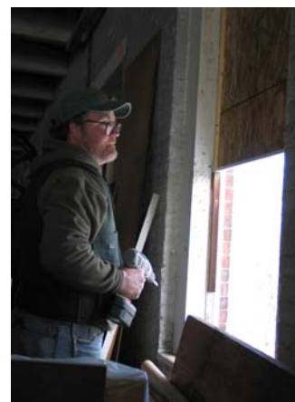
Jim Hunt returned to the museum in early February to remove the second batch of sash. Here he is protecting the window openings with plywood.
