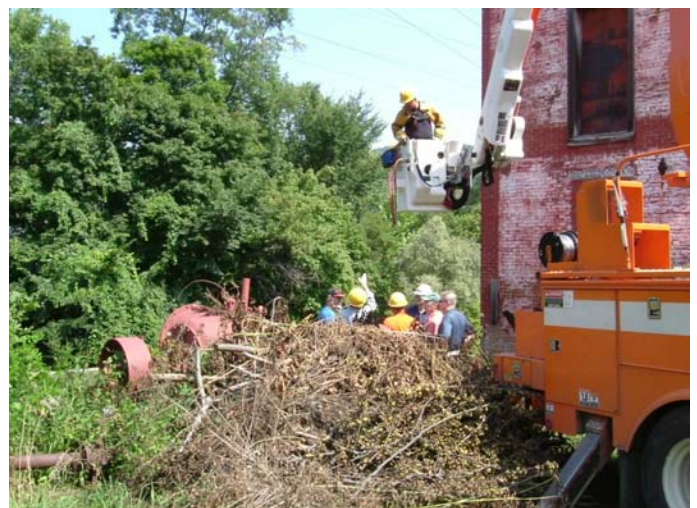
In July 04, CVPS brought a lift truck to examine the wire situation up close, with museum trustees, staff, architect Keefe and representatives from the Melanson Co., who have been awarded the roofing contract.
