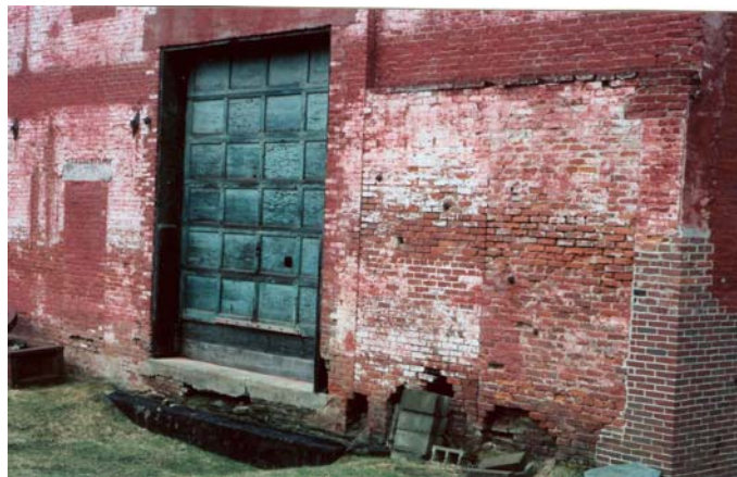
The west wall shows deteriorated mortar, poorly matched brick infill and areas of missing brick.
