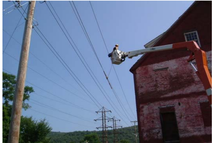
Wires from the CVPS substation behind the Armory that pass too close to the building must be moved to make it safe for the roof and windows project.
