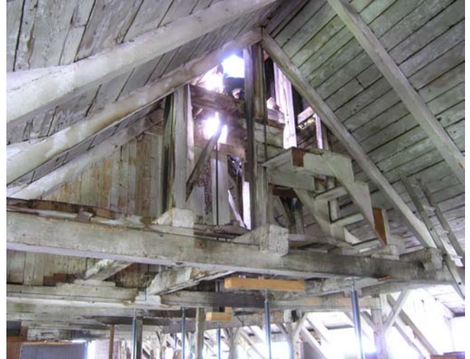
Above, temporary columns and cribbing support the attic framing. These are some of the structural issues to be addressed in the next project. Photo Tom Keefe.
