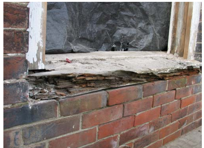
Below, this north facing window got a new sill in 2005. Many more in similar condition still need restoration. Photo John Alexander.
